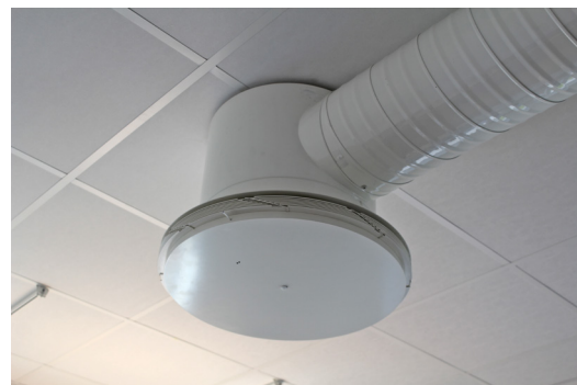
Visible mounting of the active supply air diffuser TTC with plenum box HTR.
